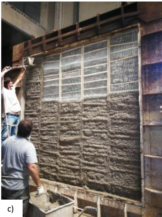
Figure 1 a) Works with the manual press activated by pulley. b) Pile of compacted plastic bottles. c) Dimensions and distribution of the wooden slats containing the plastic molds and the application of cementitious plaster. Source: Own elaboration.
